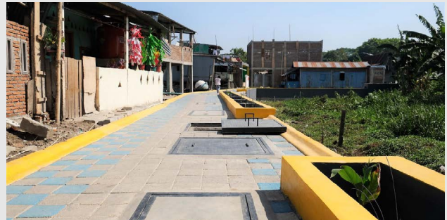
Water and sanitation intervention for a neighbourhood in Makassar comprising below-ground tanks for temporary storage, and septic tanks and constructed wetlands for sewage treatment. The intervention also included a raised pathway and drainage.
